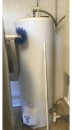
water heater Le Pradel
